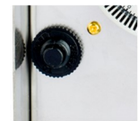
Magnetic circuit breaker on secondary to protect lighting system
